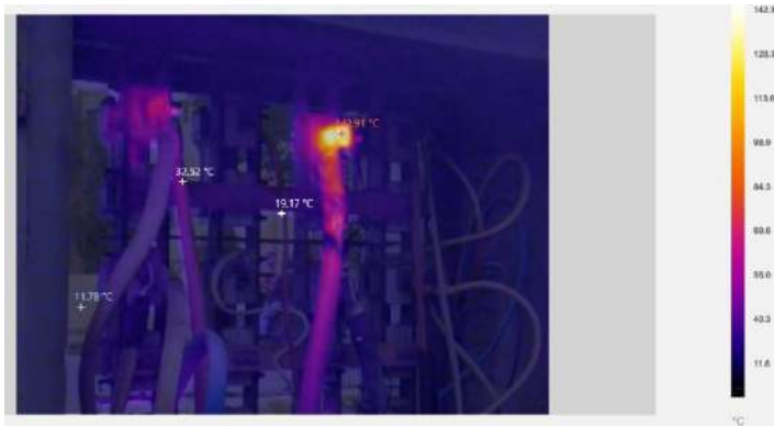
630KVA Transformer Main Incomer cable Termination
