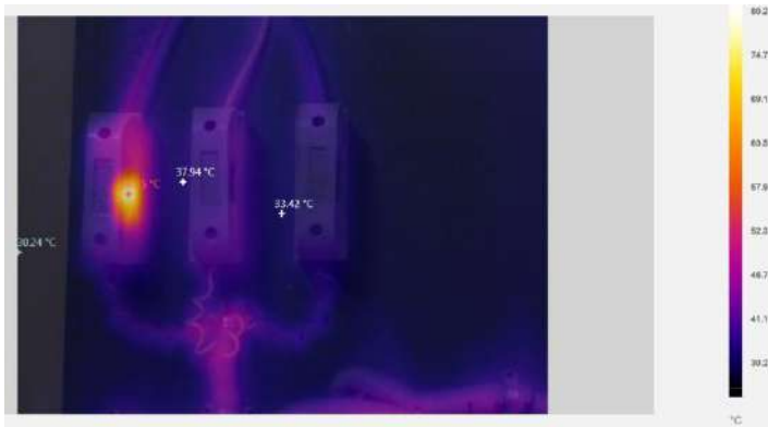
Fuse unit of the 25HP Submersible Pump
